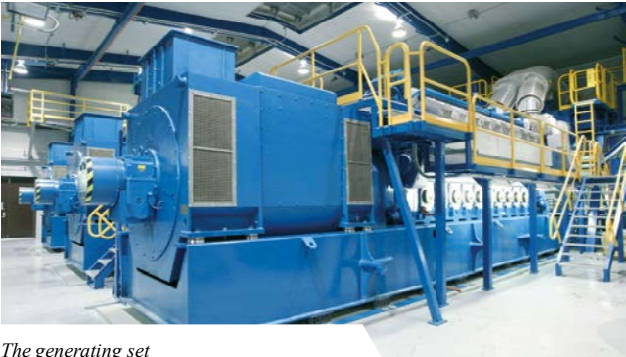
The generating set
