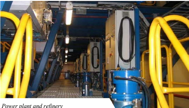
Power plant and refinery
